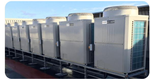
VRV Cooling System
